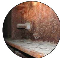
Rust and Corrosion
